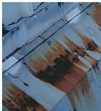
Rust and corrosion.
